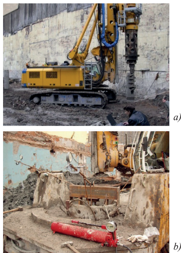
Figure 5. The complex science investigations on the construction site: taking vibration measurements during the construction of drilled cast-in-situ piles (a); the stamp test of the soil on the bottom pile's level (b).
