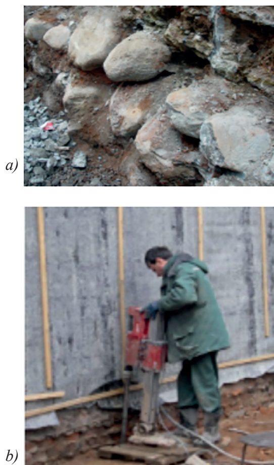
Figure 4. Underpinning of foundations and ground bed of building in Stremyannaya Street (a and b)
